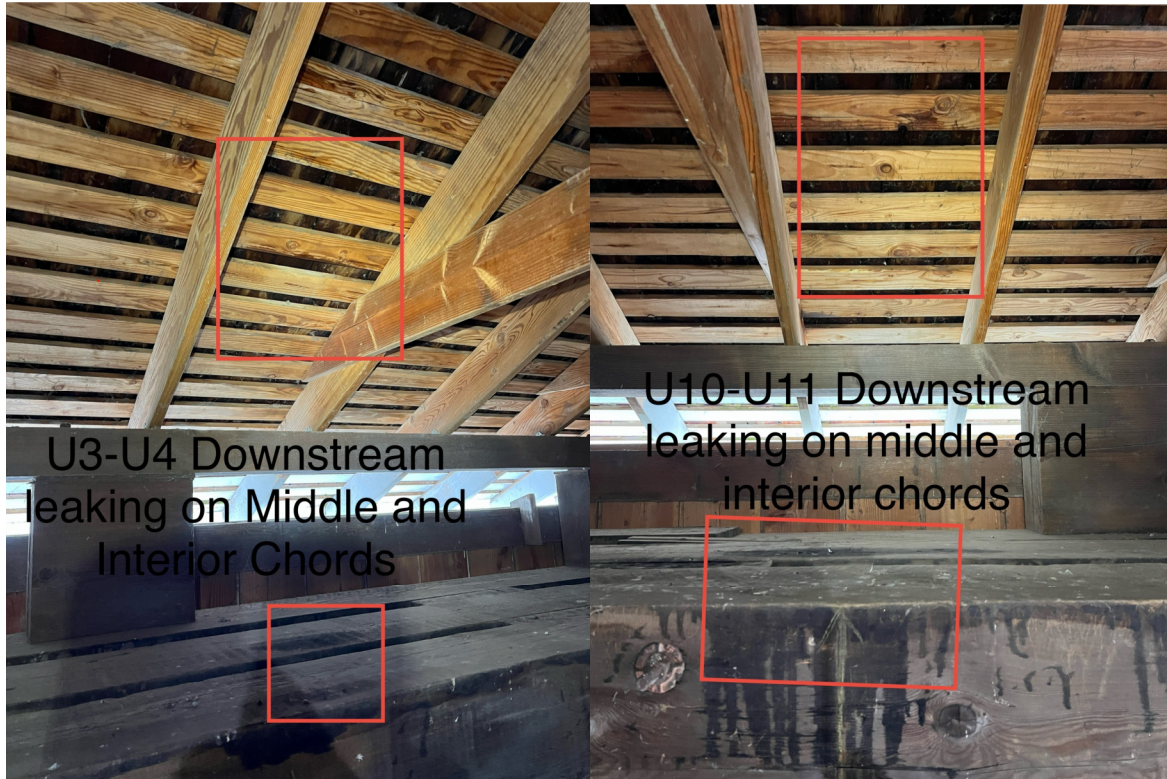
Leaks in Roof over Downstream Top Chord
