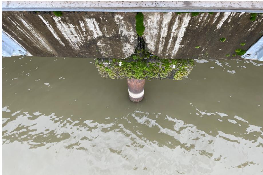
End of Slab Spalls
