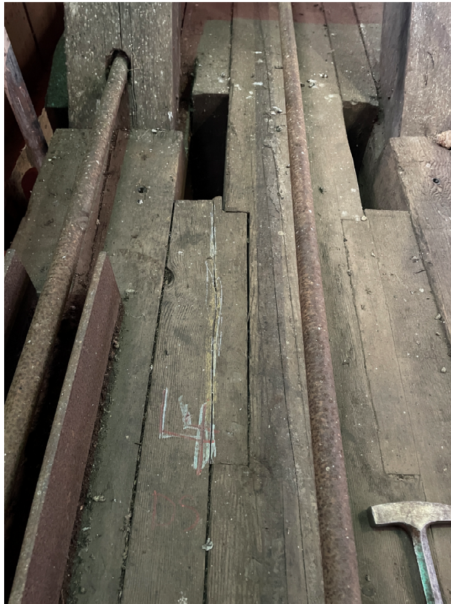
Broken and Displaced Splice in Bottom Chord near L4
