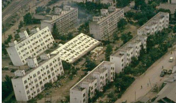
Liquefaction during the 1964 Niigata M7.6 earthquake, Honshu, Japan caused major foundation failure in these apartment blocks. Image from WikiCommons.
