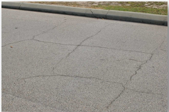
Figure 3-4 Block Cracking (not in Lowell)
