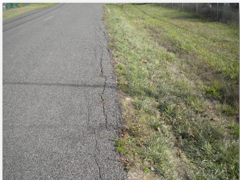
Figure 3-2 Edge Cracking on 2 nd St.
