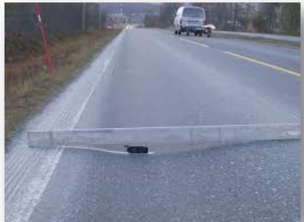
Figure 3-6 Pavement Rutting (not in Lowell)
