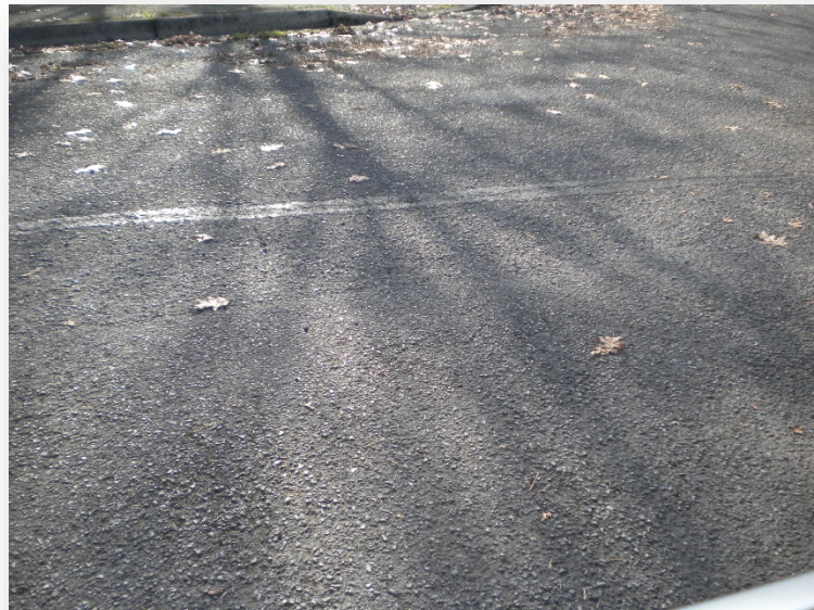
Figure 3-5 Pavement Raveling on Loftus Ave.
