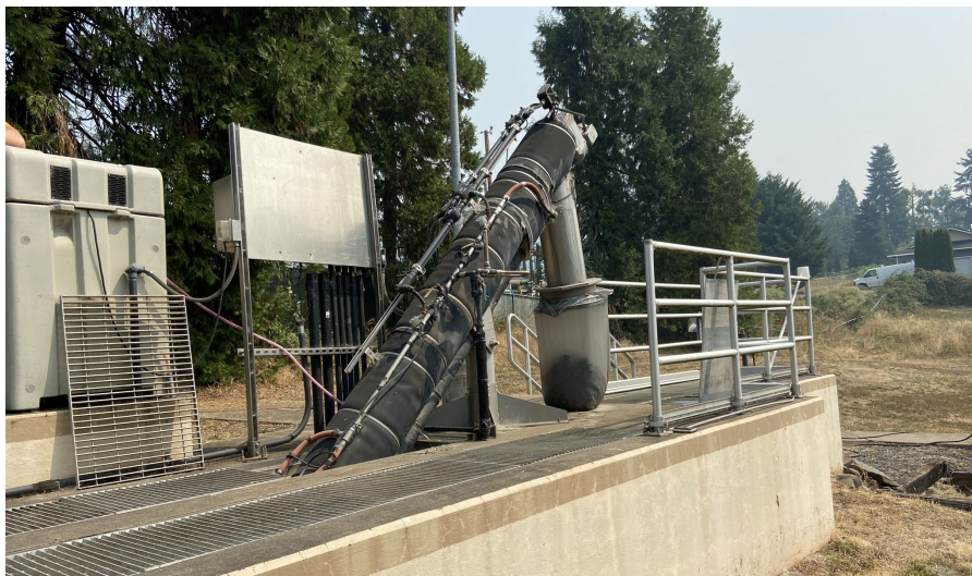
Figure 2-7: Inclined Fine Screen
