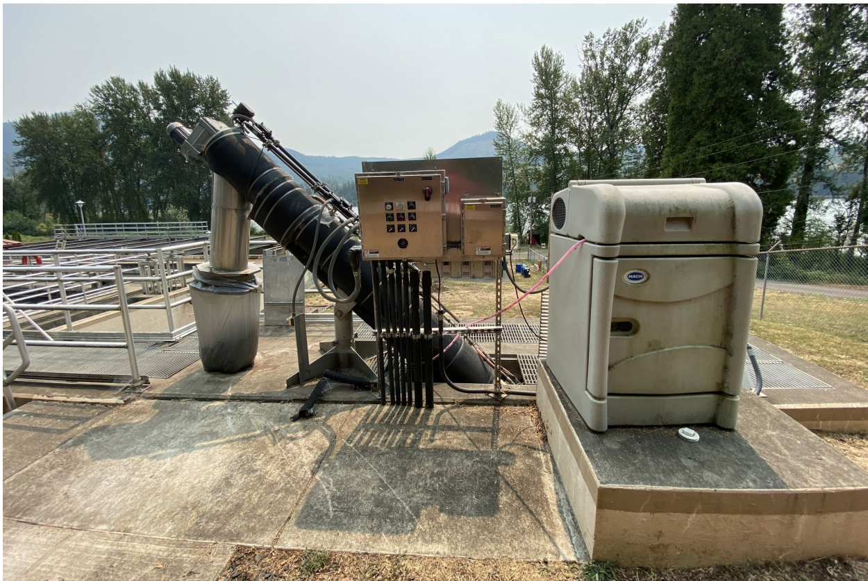
Figure 2-8: Influent Sampler and Fine Screen Control Panel
