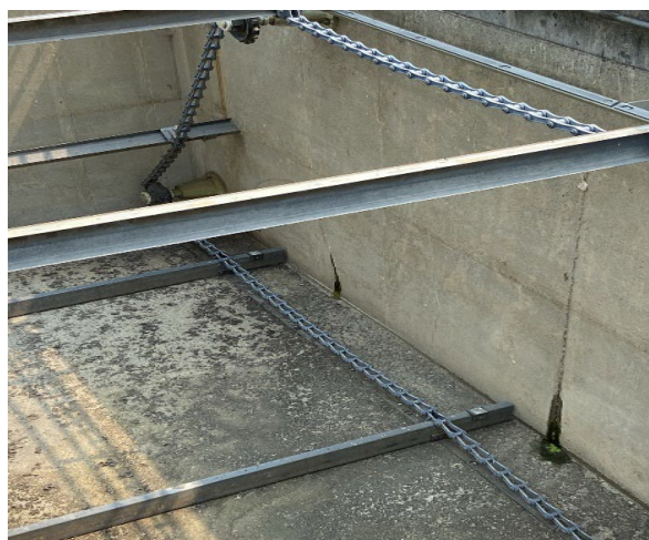
Figure 3-4: Small Cracks in Clarifier Wall
