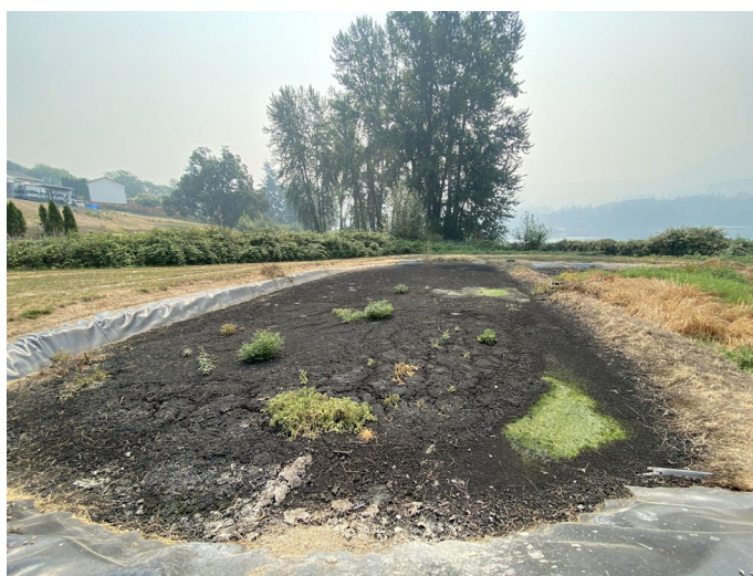
Figure 2-13: Eastern Sludge Drying Bed
