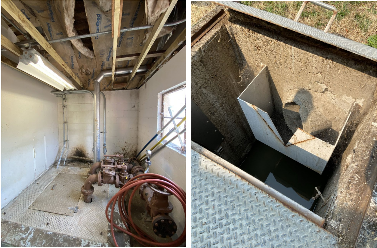
Figure 2-2: Alder Street Pump Station Wetwell and Intake (Left) and Emergency Overflow and Weir (Right)
