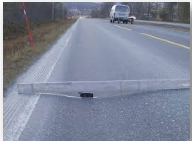
Figure 3-6 Pavement Rutting (not in Lowell)
