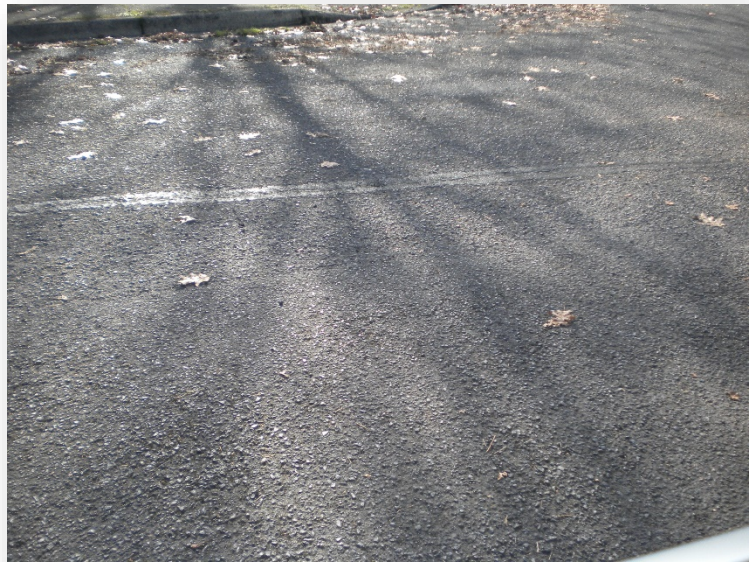
Figure 3-5 Pavement Raveling on Loftus Ave.
