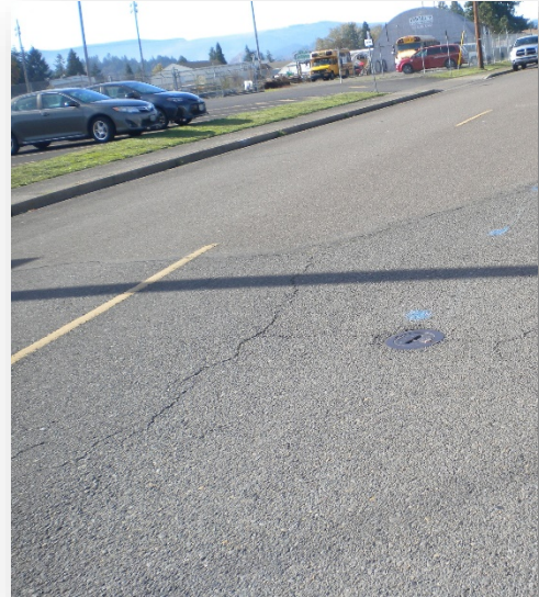
Figure 3-3 Longitudinal Cracking on Main St.
