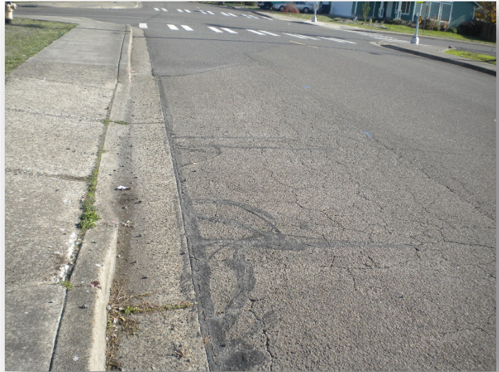
Figure 3-1 Alligator Cracking on Main St.
