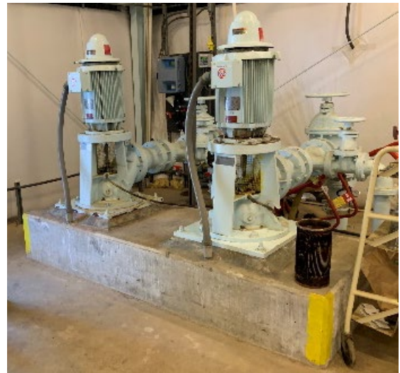
PHOTO 7.2.3 – FINISHED WATER PUMPS
