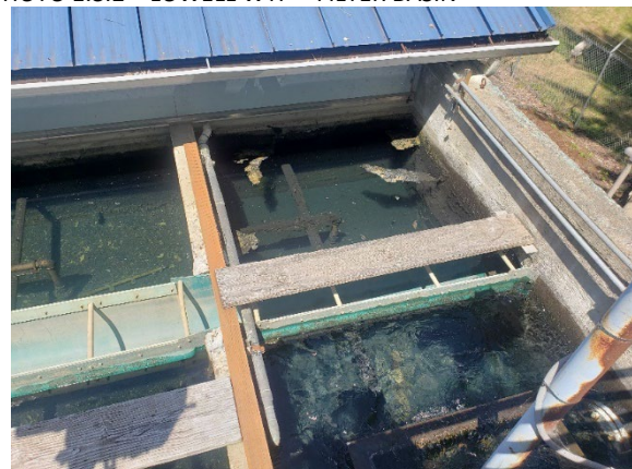
PHOTO 1.3.2 – LOWELL WTP – FILTER BASIN
