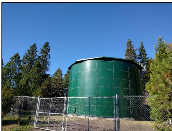
The City of Lowell maintains two above ground storage tanks with a combined capacity of just over 1,000,000 gallons.
