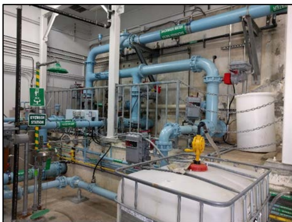
Interior of the Water Treatment Plant
